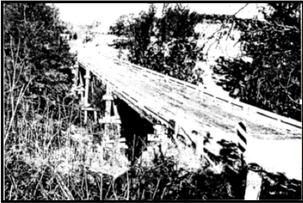
Cuneens Bridge built by the Keever brothers in 1895/6 with Patrick Cuneen's land grant in background. (Photo: E. Roberts)
