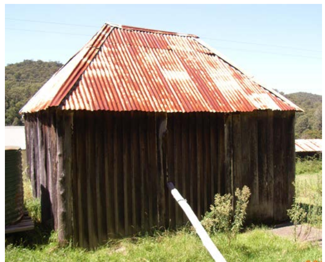
Slab hut Murrays Run Road at Bucketty, repaired with sawn timber and cover strips to keep the wind out and with a tin roof. Note Flea Bane in full seed in front of hut.
