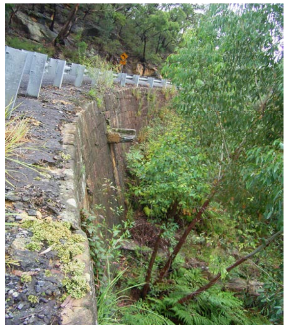
Wall and culvert lip at Ramsays Leap showing sheer drop
