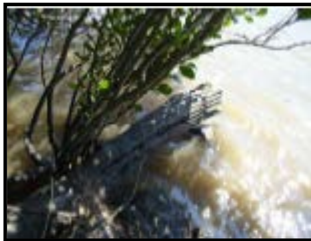
Wharf timber with scarf cut in near front end Photo E. A. Roberts
